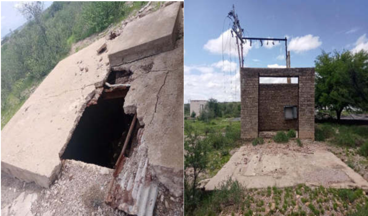
(Left) Vandalized underground tunnel at waypoint 179. (Right) A remnant of a structure used for electrical facility.
