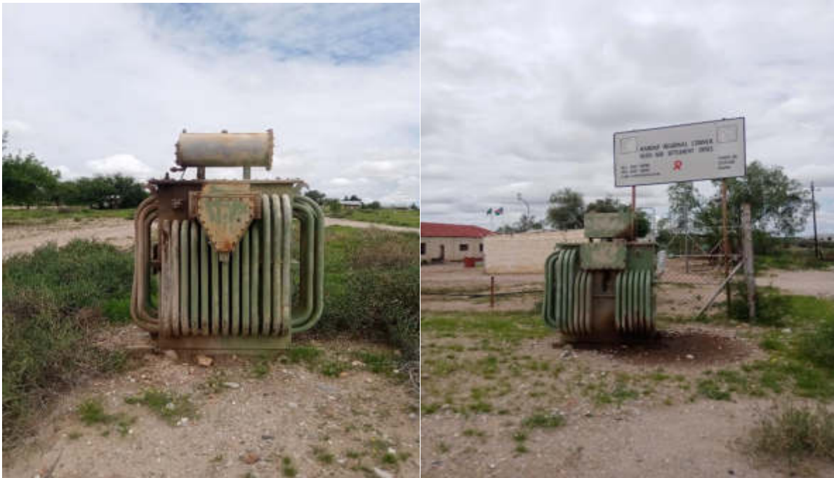
Old transformers that used to provide electricity for copper mine
