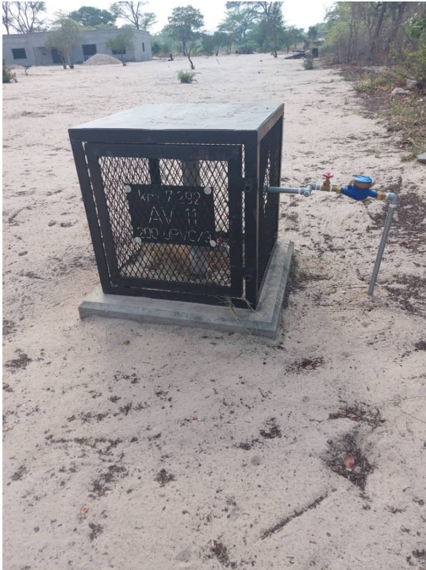
Figure 7: installed and existing rural water supply pipeline katima sibbinda along the project area
