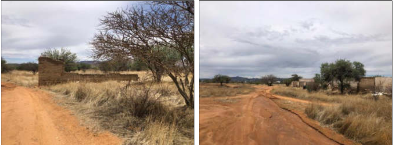
Figure 4: Existing dilapidated infrastructure
