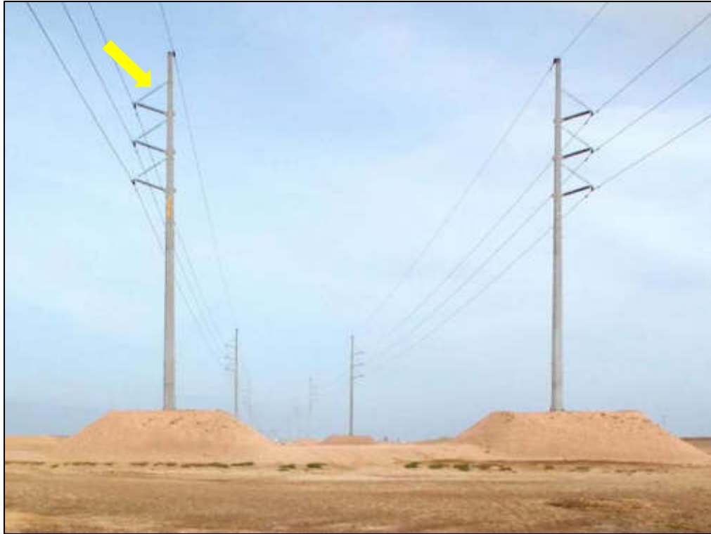
Figure 37. Example of a braced/slanting insulator, where the slope of the insulator may discourage perching by large birds such as vultures, used as a mitigation for electrocutions on the 132 kV steel monopole Kuiseb-Walvis Bay power line.
