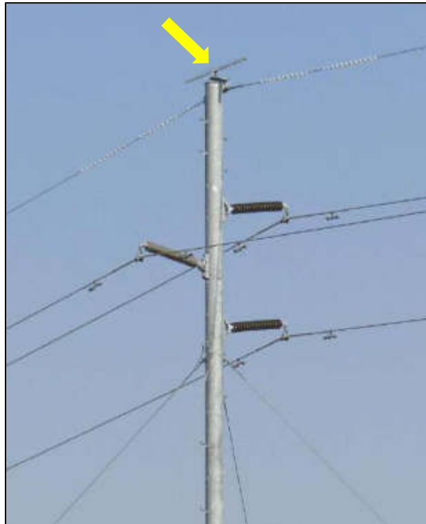
Figure 36. Example of an inexpensive bird perch device, used in order to encourage vultures and other raptors and large species to perch at the top of the tower structure, rather than on the insulators, as a mitigation for bird electrocutions on the 132 kV Auas-Naruchas power line.
