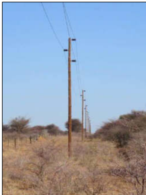
Figure 7. An existing Cenored 33 kV distribution line on Farm Lardner.
