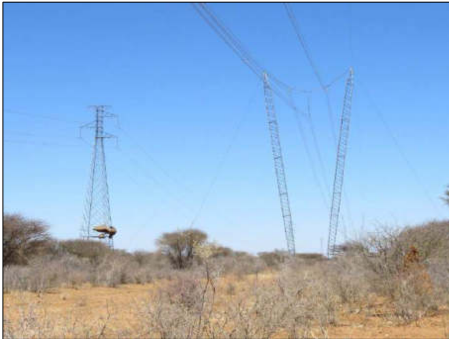
Figure 6. The existing NamPower 220 kV Gerus-Otjikoto line (No. 1 and 2) on Farm Maxwell (looking south-westwards), consisting of a self-support steel lattice structure (left) and a guyed-V structure (right). Note the large Sociable Weaver nest on the left-hand tower.
