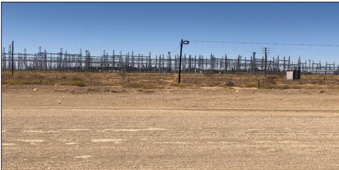
Figure 4: NamPower Kokerboom Transmitter Station (2)
