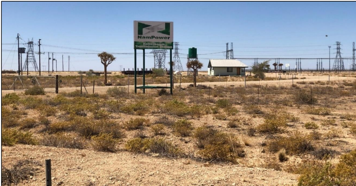
Figure 3: NamPower Kokerboom Transmitter Station (1)
