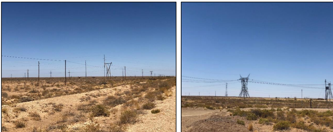
Figure 13: Various powerlines from and to the Transmitter Station
