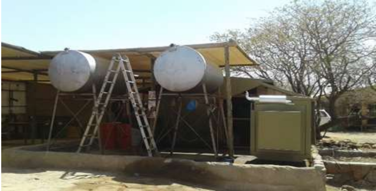
Figure 8: Workshop and diesel storage tanks
