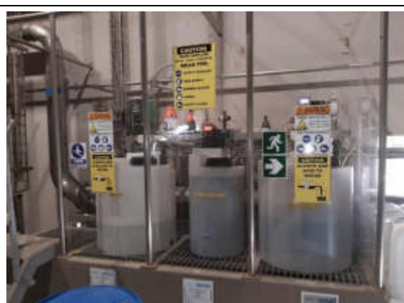
Photo 4-7. Water treatment facilities
