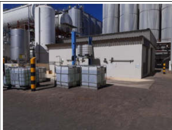
Photo 4-26. Chemical storage area
