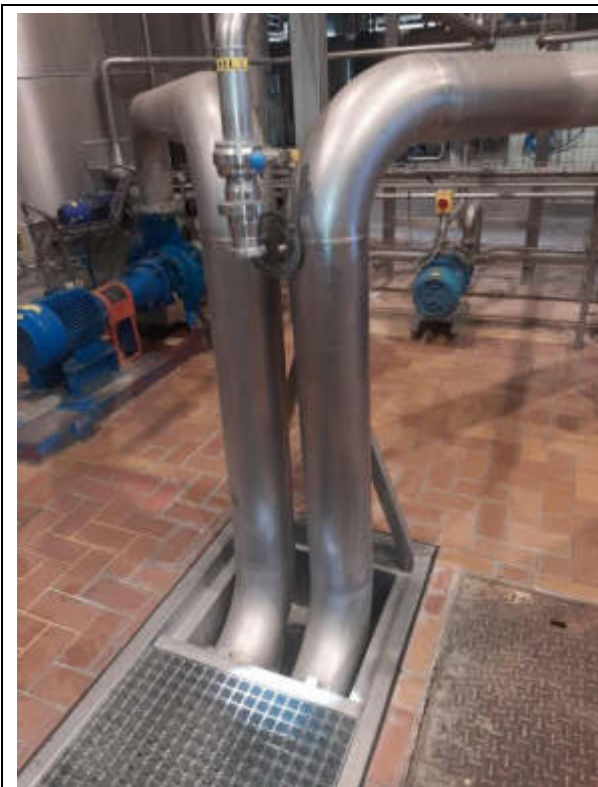
Photo 4-22. Effluent pipes from brewing process
