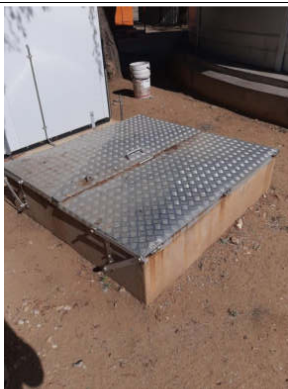
Photo 4-23. Effluent sampling point
