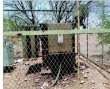
DAMAGES: At least 40 houses have been affected by an electrical blunder which stretched over three streets in Damara location. PHOTOS: ESTER KAMATI
