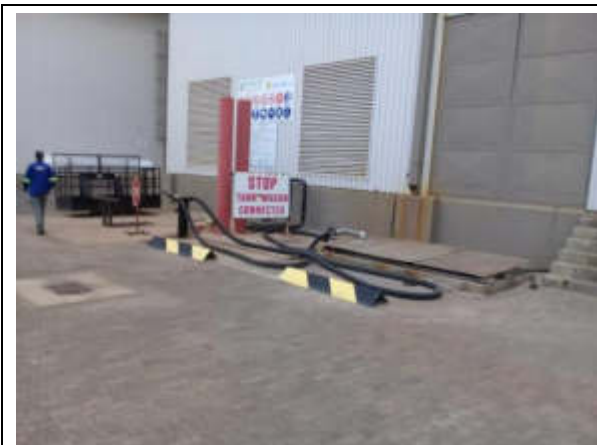
Photo 4-14. HFO offloading point
