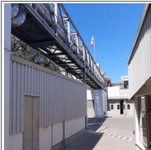
Photo 4-20. Ammonia storage shed and overhead pipe trestle
