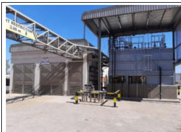
Photo 4-6. Water treatment plant
