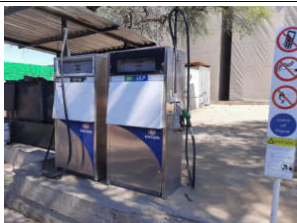
Photo 4-16. Consumer fuel installation
