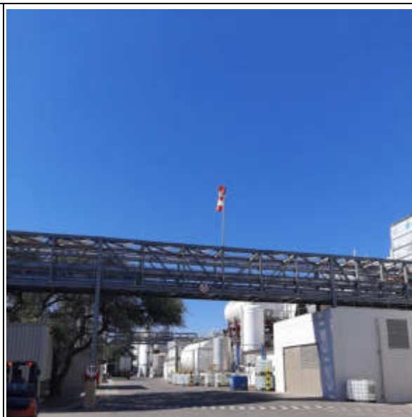
Photo 4-21. Ammonia pipe trestle with wind cone
