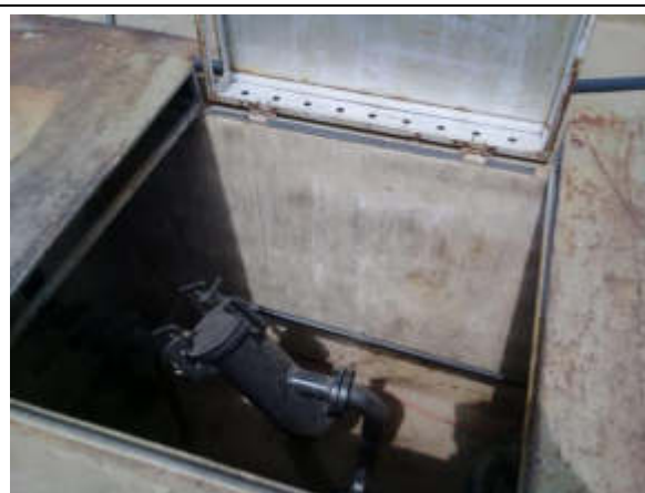
Photo 4-15. Underground HFO reticulation
