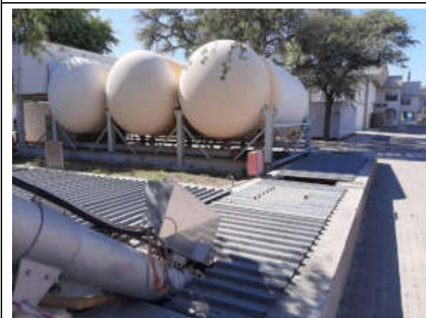
Photo 4-24. Effluent screening infrastructure
