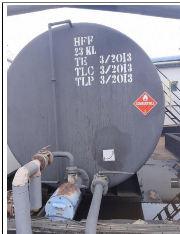
Photo 4-14. HFO tank inside bund area
