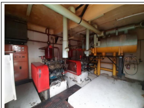
Photo 4-10. Compressor room and ammonia storage
