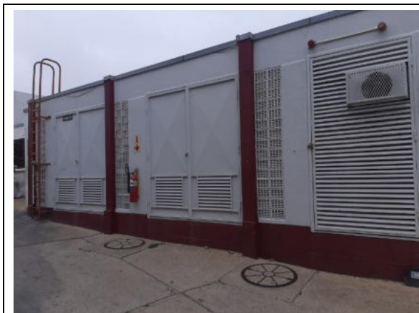
Photo 4-11. Generator room - factory
