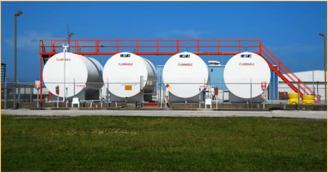
Figure 6: A typical above-ground Diesel storage, a similar is proposed by TradePort Namibia (Source: EPA, 2021)
