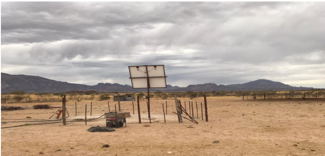
Figure 19: Solar panels recorded within EPL 8092.
