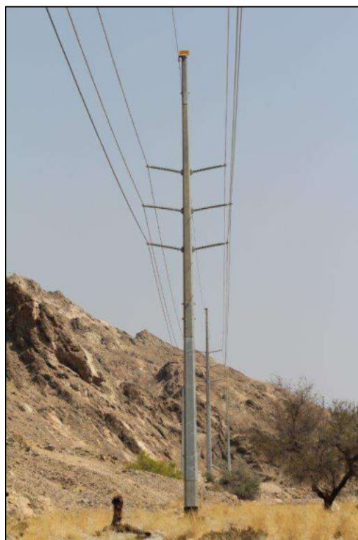
FIGURE 3: PHOTO SHOWING AN EXAMPLE OF A STEEL MONOPOLE STRUCTURE FOR THE 132 KV POWERLINE
