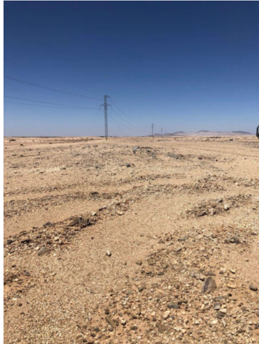
FIGURE 10: PHOTO SHOWING THE DISTURBED PARTS OF THE POWERLINE CORRIDOR
