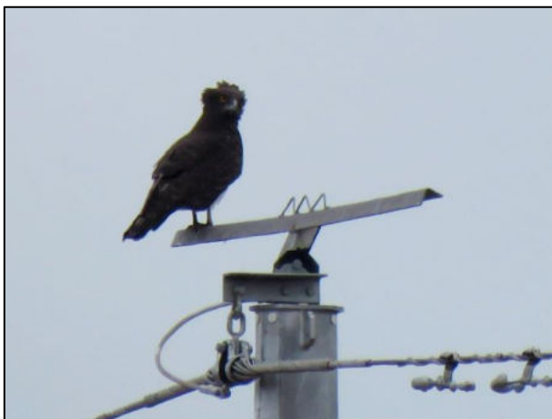
Figure 36. Example of a Brown Snake Eagle making use of a perching structure fitted to a 66 kV steel monopole.
