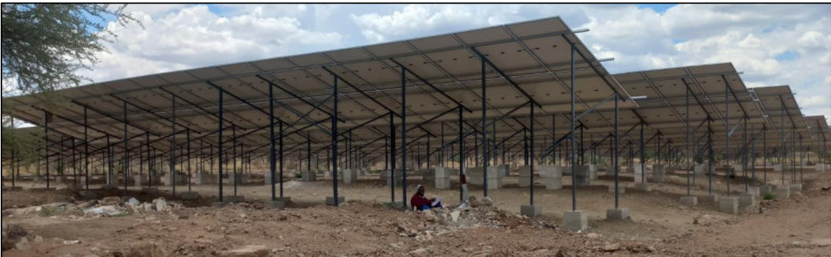
Figure 8: Solar panels on site providing electricity
