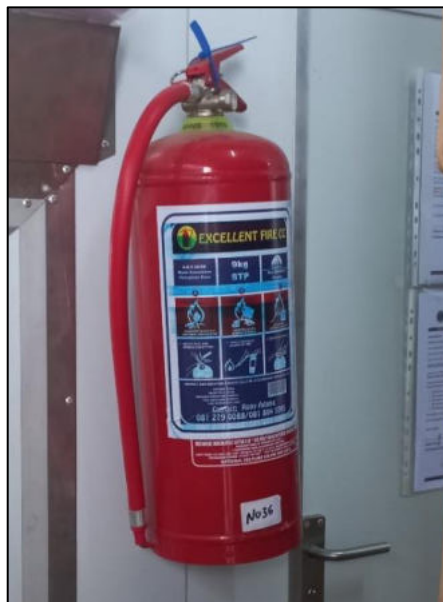
Figure 10: Fire extinguisher on site
