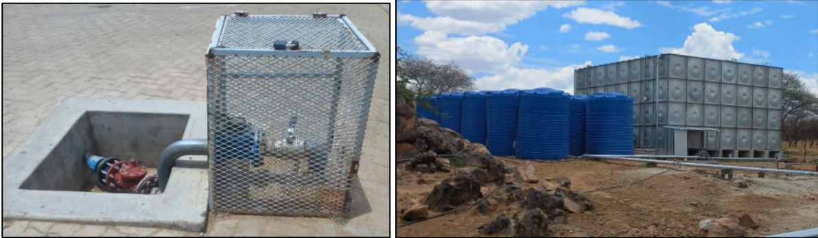
Figure 7: Water connection to site and water storage tanks on site
