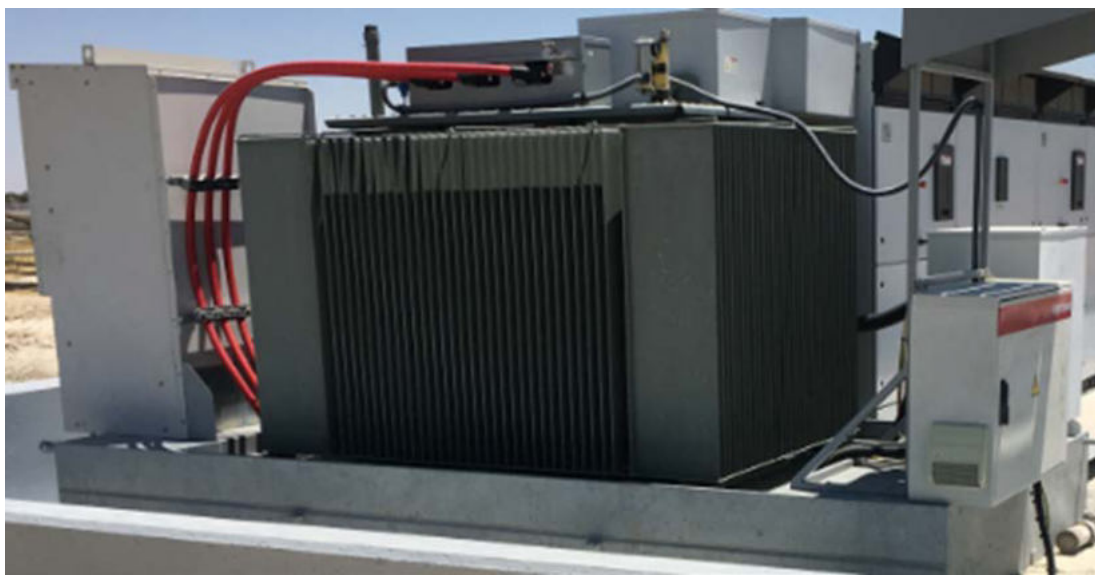
Photo 4.2 – Example of a field transformer
