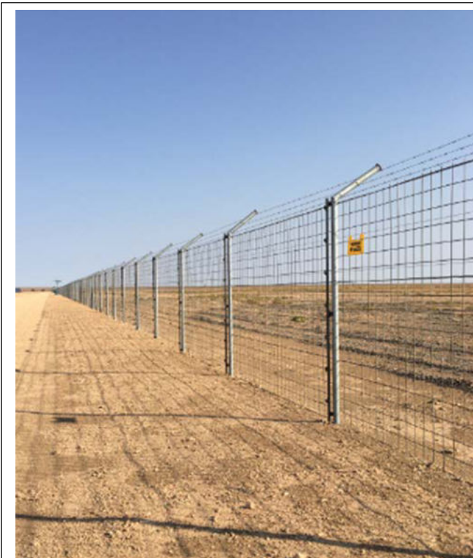
Photo 4.4 – View of a similar electrified security fence
