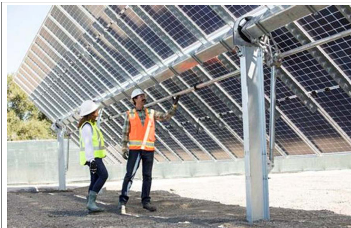
Photo 4.1 – Example of single axis tracking system
