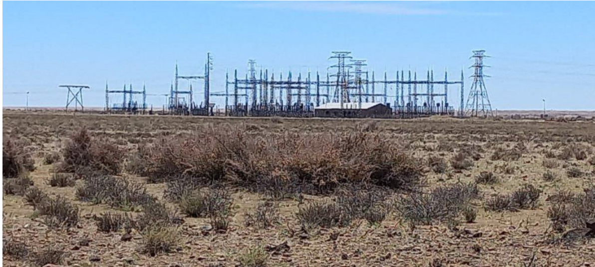
Photo 4.6 – View of Harib Substation
