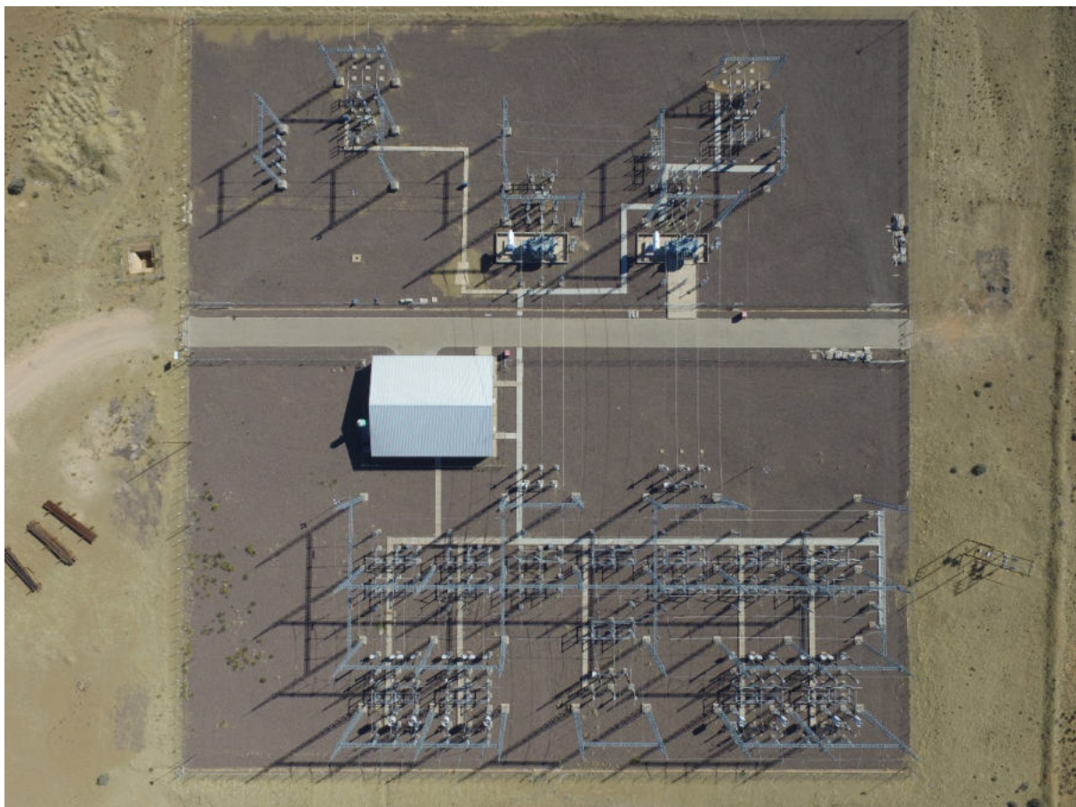
Photo 4.7 – Arial View of Harib Substation
