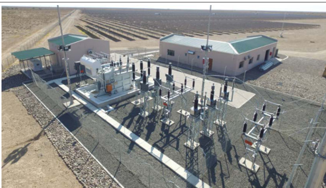
Photo 4.3 – View of a similar site substation & buildings
