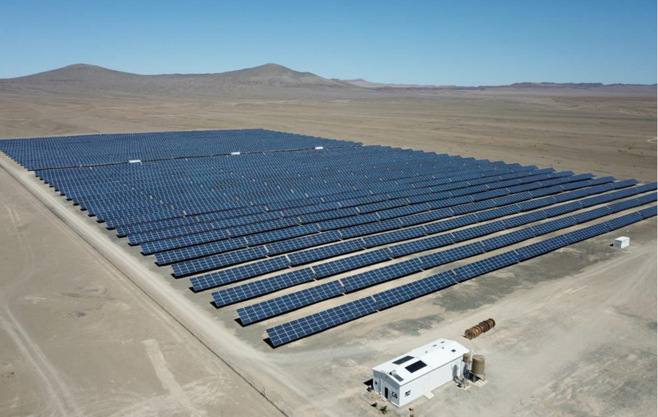
Plate 1.2: The operational Aussenkehr 5MW Solar PV Park (Source: ALCON, 2019).
