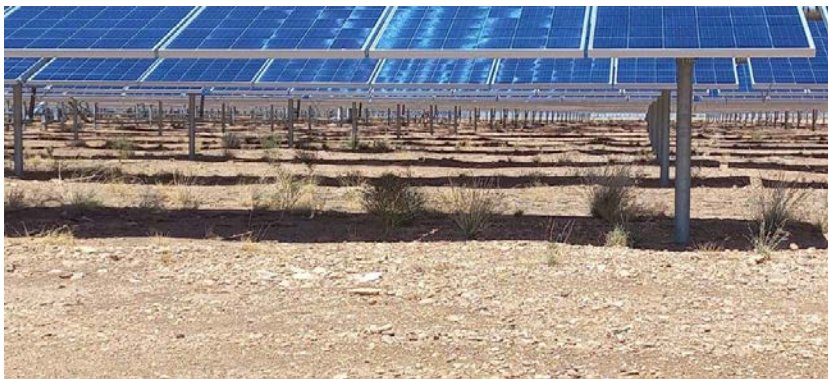
Photo 25 – View of PV panels with some ground cover vegetation.
