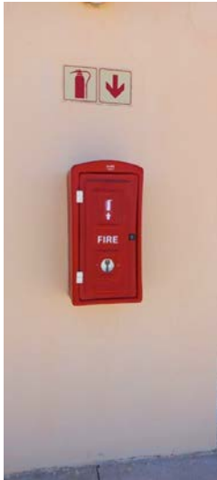
Photo 10 – View of fire extinguisher at site office.
