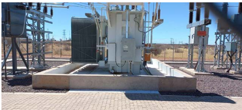
Photo 12 – View of transformer located within bunded area.
