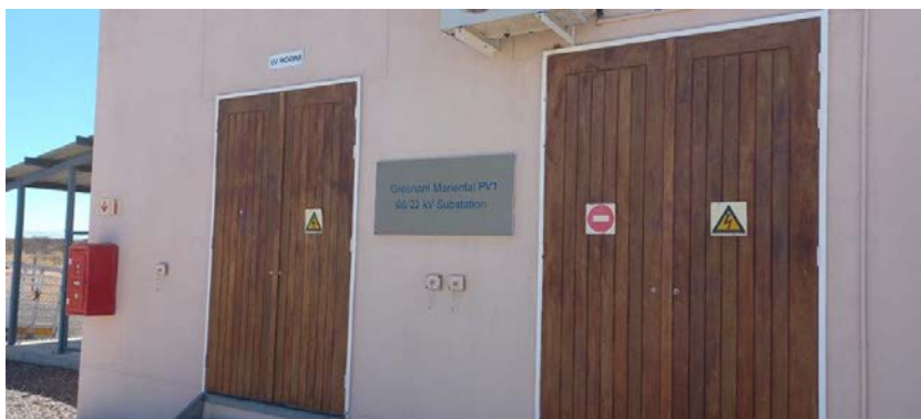
Photo 13 – View of site's substation building with fire extinguisher.
