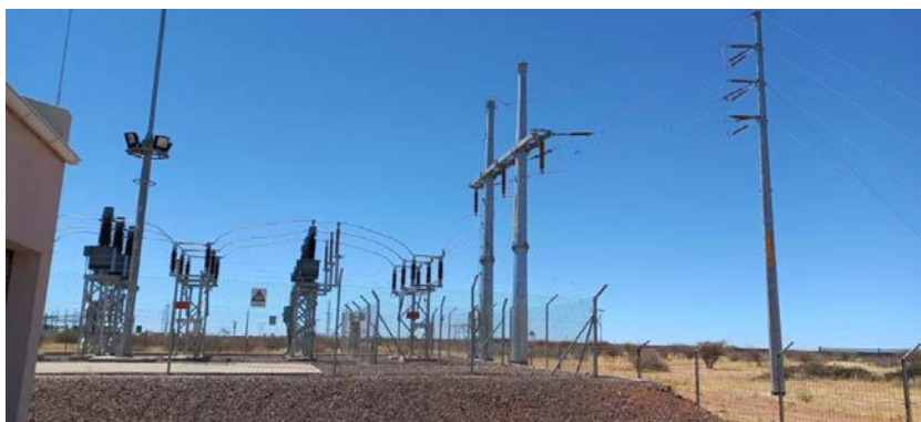
Photo 11 – View of site's substation fenced-in and well maintained.
