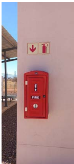
Photo 10 – View of fire extinguisher at site office.
