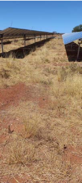
Photo 20 – View of PV panels with are having good ground cover vegetation.
