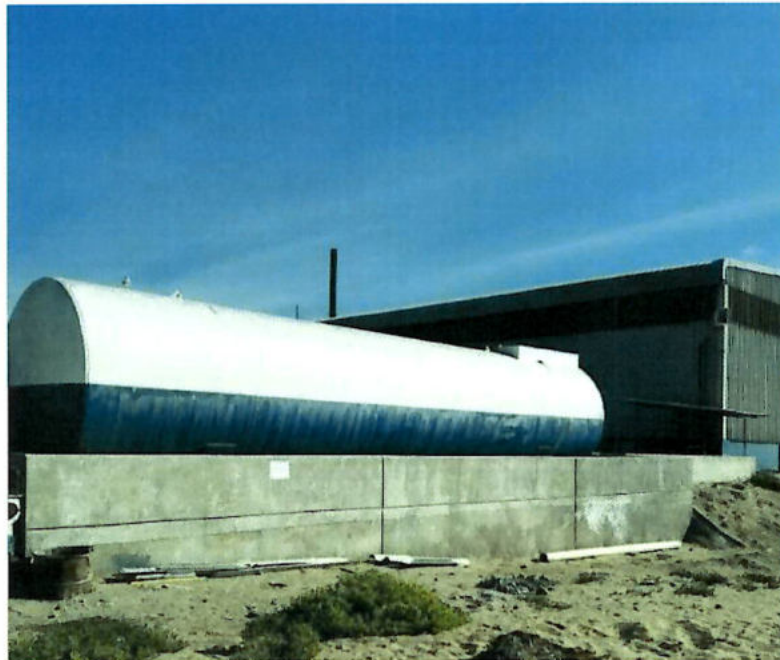
Fig 4.4.1 Fuel Oil Storage Tank
