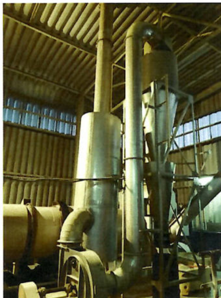
Fig 4.3.3 Scrubber with Cyclone and extractor fan
