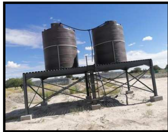
Figure 14: Overhead water storage tanks at the site
