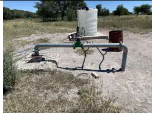
Photo 4-25 Borehole pump installation used for irrigation (EB11)
