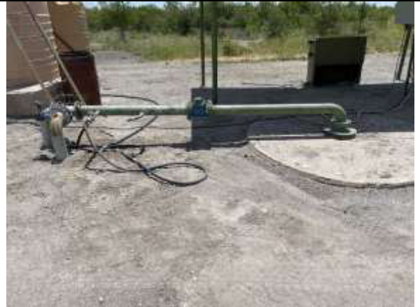
Photo 4-26 Borehole pump installation used for irrigation (WW100069 / EB7)
