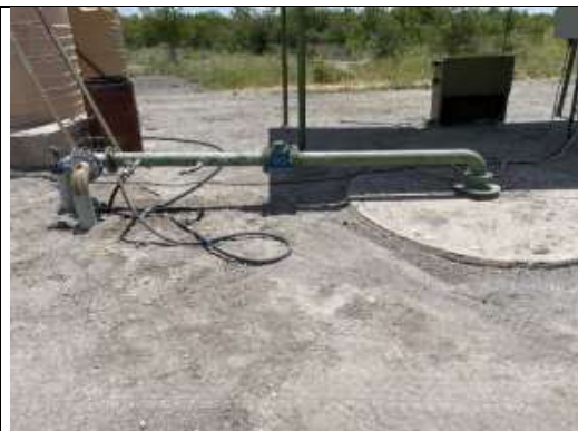
Photo 7-2 Borehole pump installation used for irrigation (WWW100069 / EB7)
