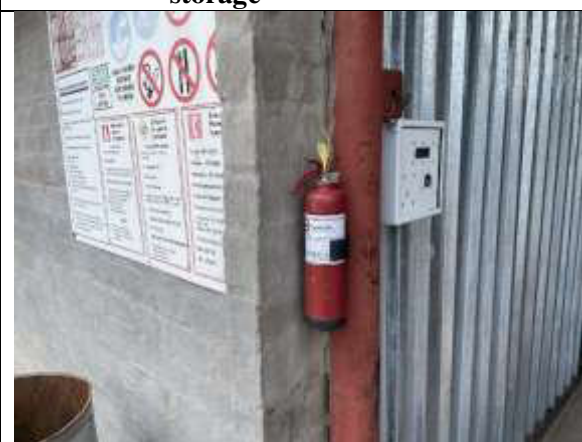
Photo 4-22 Fire hydrant and safety signs at the entrance of the shed
