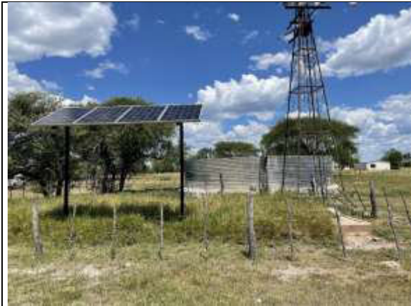
Photo 4-15 Solar panel used at boreholes
