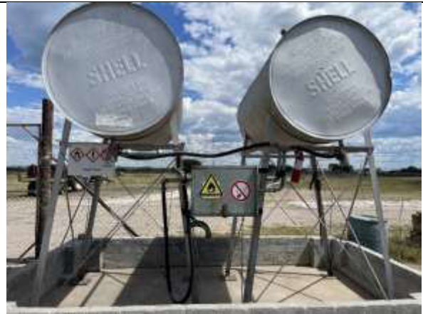
Photo 4-16 Fuel storage tanks
