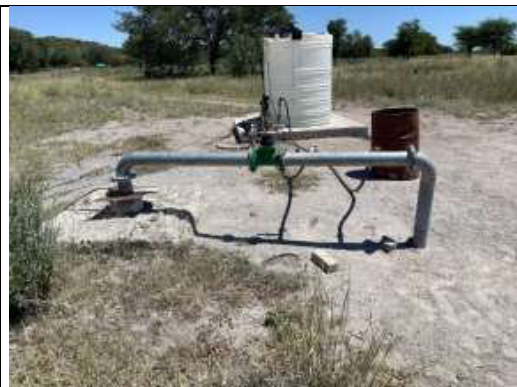
Photo 7-1 Borehole pump installation used for irrigation (EB11)
