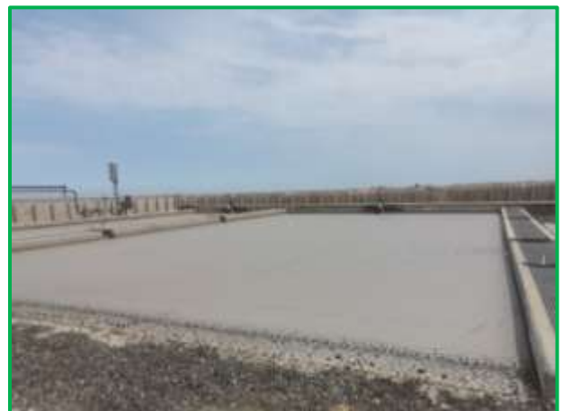
Figure 9: Sludge in the dry pond
