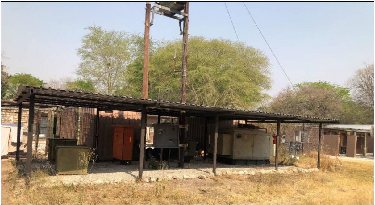
Figure 8: Electricity facilities on site
