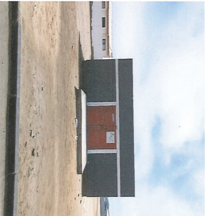
Picture indicates the Electrical Substation of Erf 504, Tamariskia, Ext No. 1
