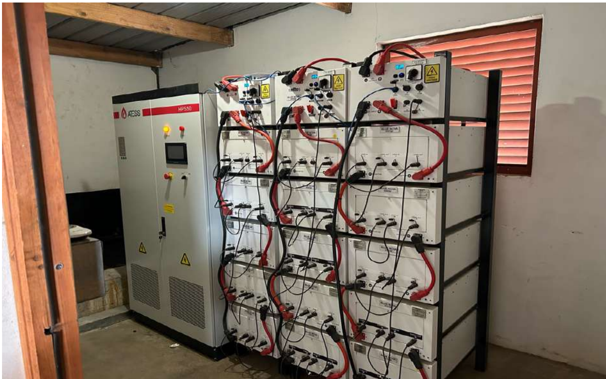
Figure 6 Lodge: Generator Building BESS
