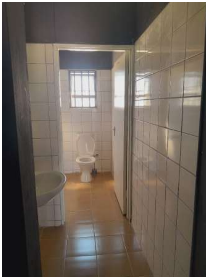
Figure 2-8: One of the two flushing toilets at the Namfocus Service Station
