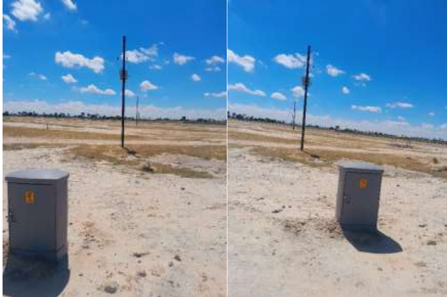
Figure 2-5: The NORED power lines near the site
