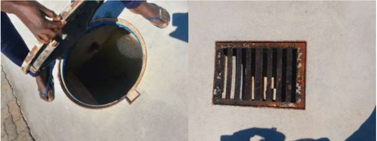
Figure 2-7: Oil-water separator structures onsite
