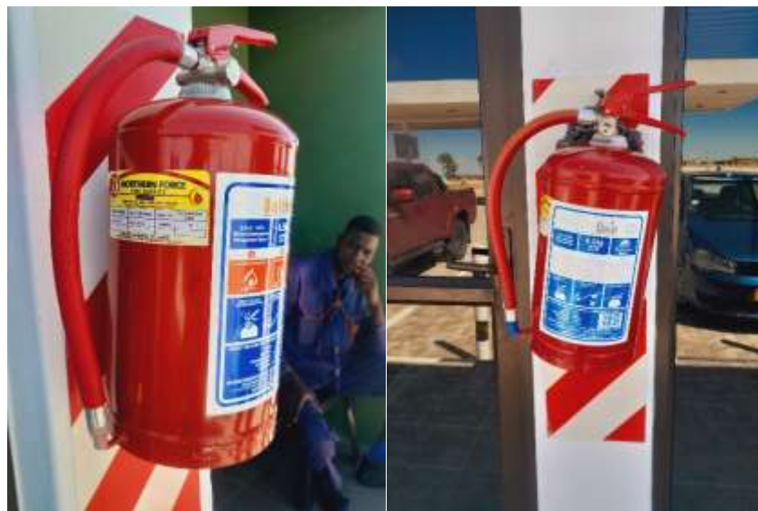
Figure 2-10: One of the four fire extinguishers onsite
