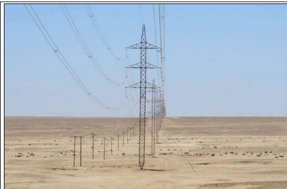
Photo 4.4.2 – Existing two 220 kV and 22 kV transmission lines north of Walmund Substation (viewed south to north)
