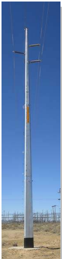
Photo 4.5.1 - View of single-circuit freestanding monopole structure
