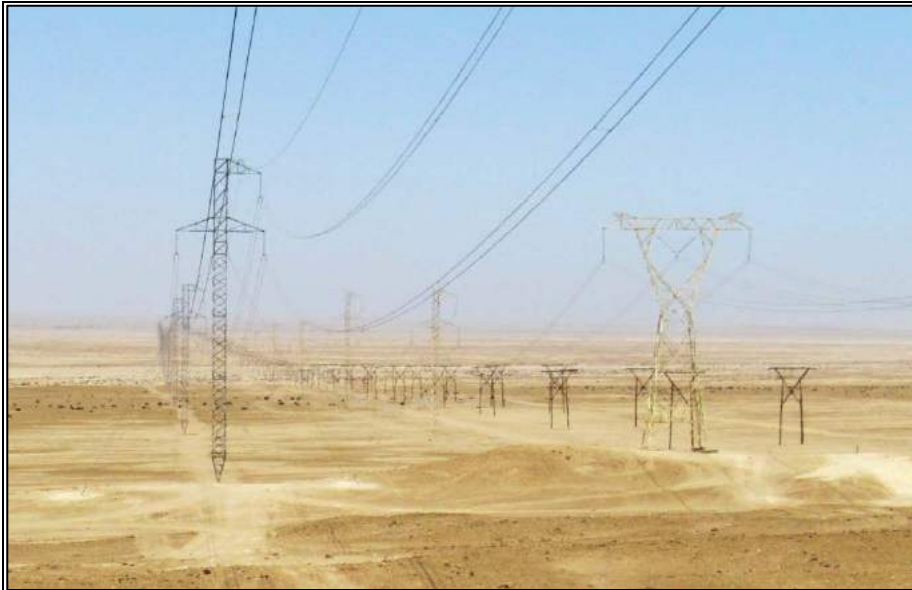
Photo 4.4.1 – Existing two 220 kV and two 66 kV OHTL between Kuiseb and Walmund Substations (viewed north to south)
