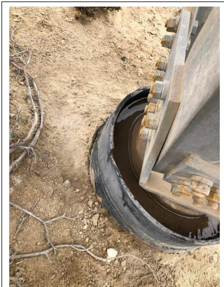
Photo 7.4.1 – Water forms at the base of the OHTL from fog that condensate on the steel structures
