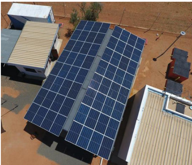
Figure 3 Solar PV Plant
