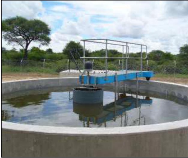
Figure 19: Clarifier with Rotating Bridge
