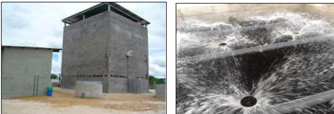
Figure 22: Trickling Tower with Wetting (Spray Nozzles) on Top
