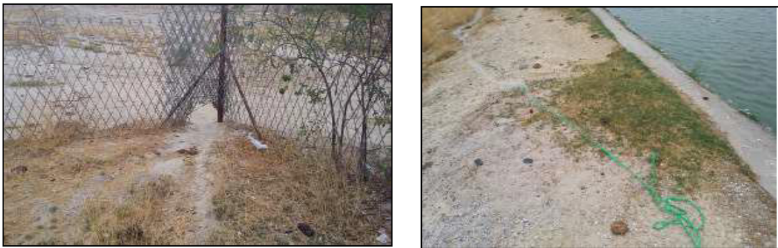
Figure 8: Oshakati West Ponds – damaged fence and evidence of fishing activities
