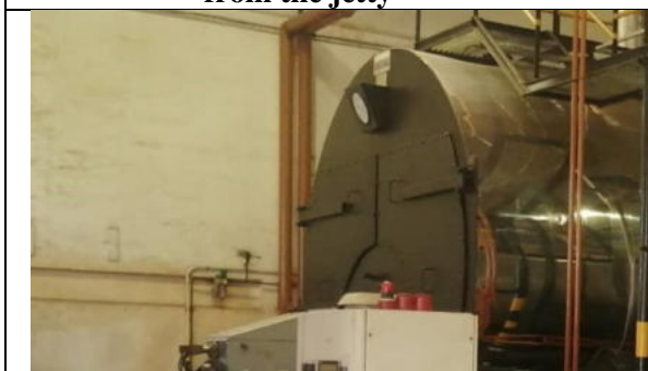
Photo 2-3 Fishmeal and cannery plant 20 t boiler
