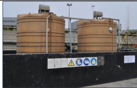
Photo 2-6 Ultra Floc solution and 3TL Sud Floc on site storage tanks
