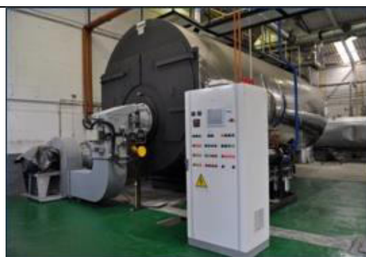
Photo 2-2 Fishmeal and cannery plant 10 t boiler
