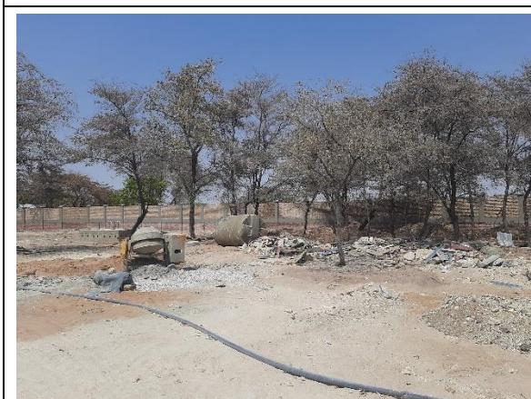
Photo 4-4. Consumer installation site (photo 2)
