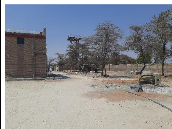
Photo 4-3. Consumer installation site (photo 1)
