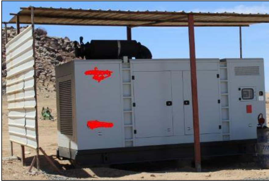
Figure 2-3. Typical overhead shaded structure installed over a diesel engine powered generator mounted to a concrete slab
