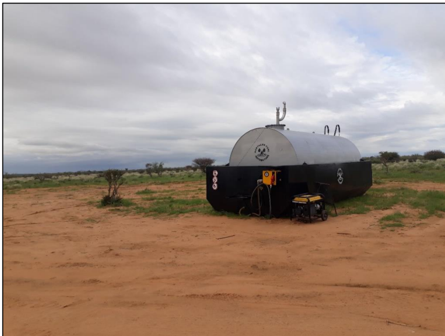
Figure 2-2. An example of a 10 000L diesel tank installed onsite for diesel storage
