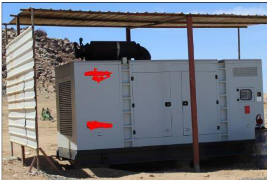
Figure 2.3. Typical overhead shaded structure installed over a diesel engine powered generator mounted to a concrete slab
