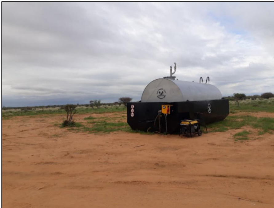
Figure 2.2. An example of a 10 000L diesel tank installed onsite for diesel storage
