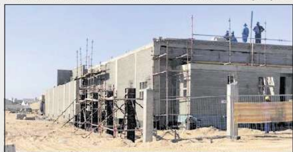
The Paratus landing station will host the Equiano undersea cable system transmission equipment.
