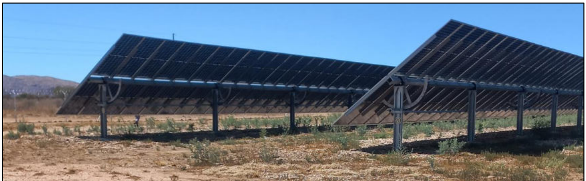
Figure 12: PV Plant on site
