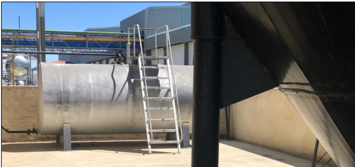
Figure 8: Diesel storage facilities (2)
