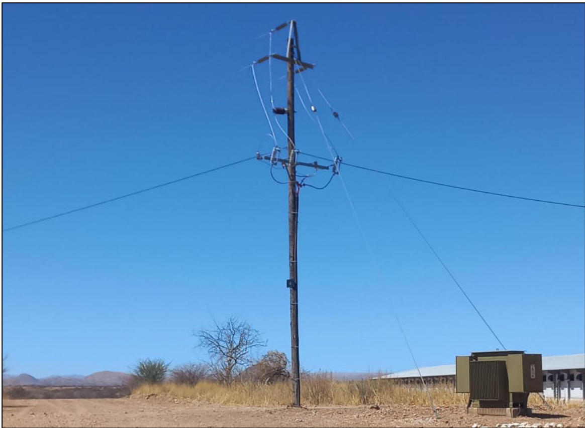
Figure 11: Electricity to site
