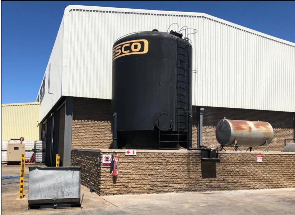
Figure 7: Diesel storage facilities (1)
