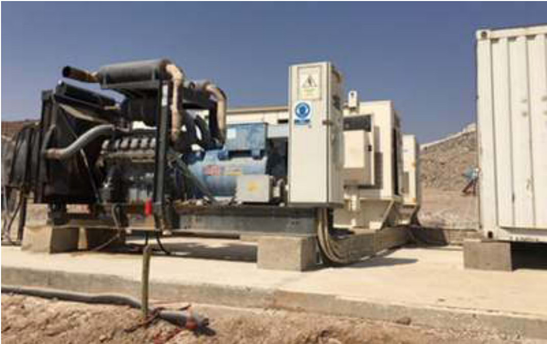
Figure 10 - Genset stand-by power source (Source: Minxcon, 2021)
