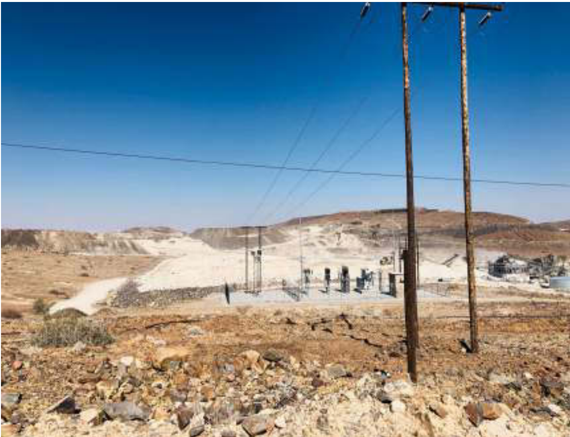
Figure 9 - Main power supply off take (Source: ECC, 2021)
