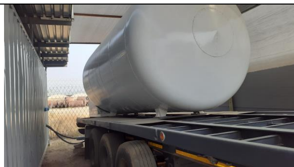
Photo 2. Mobile CO 2 tank
