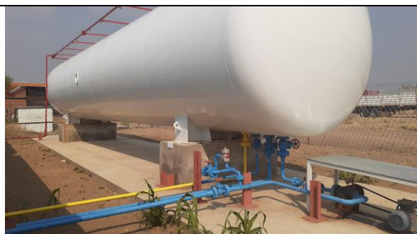
Photo 1. LPG Storage tanks with Fire Protection
