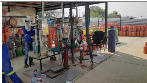
Photo 4. Gas Cylinder filling bay
