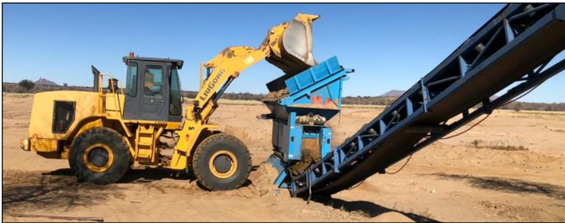
Figure 4: Screen and hopper, conveyor belt and loader
