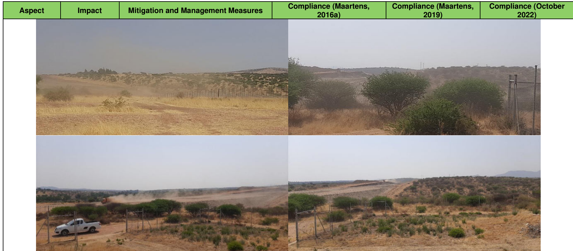
Figure 7: Pictures showing the dust (particulate matter) pollution in the area due to the construction of the new B6 road (Source: L. Maartens, 12 October 2022).
