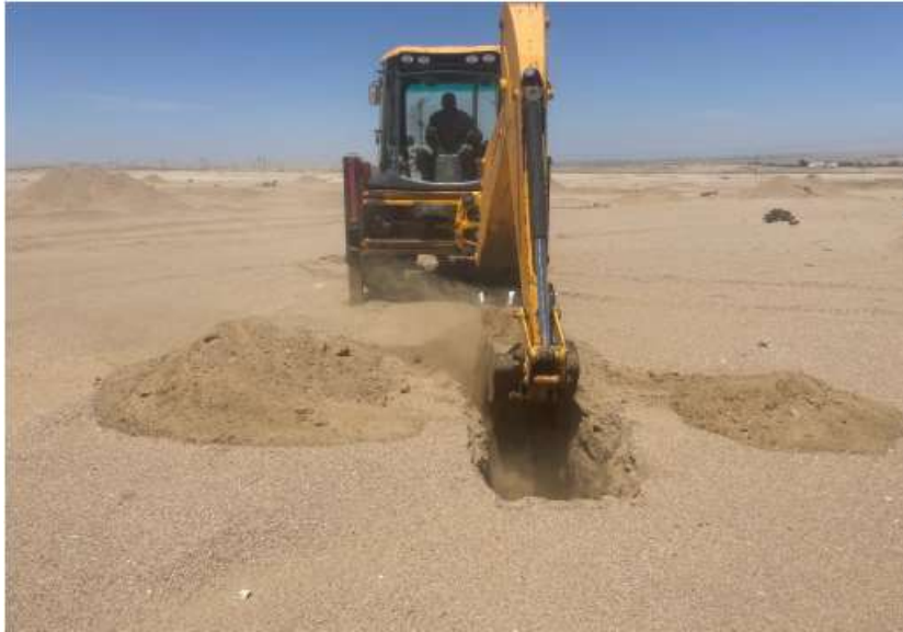
Picture 14 Test pits dug up to examine the soil profiles during geotechnical assessment in the focus area.
