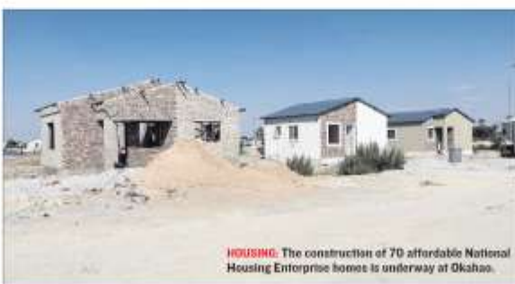
HOUSING: The construction of 70 affordable National Housing Enterprise homes is underway at Okahao.
