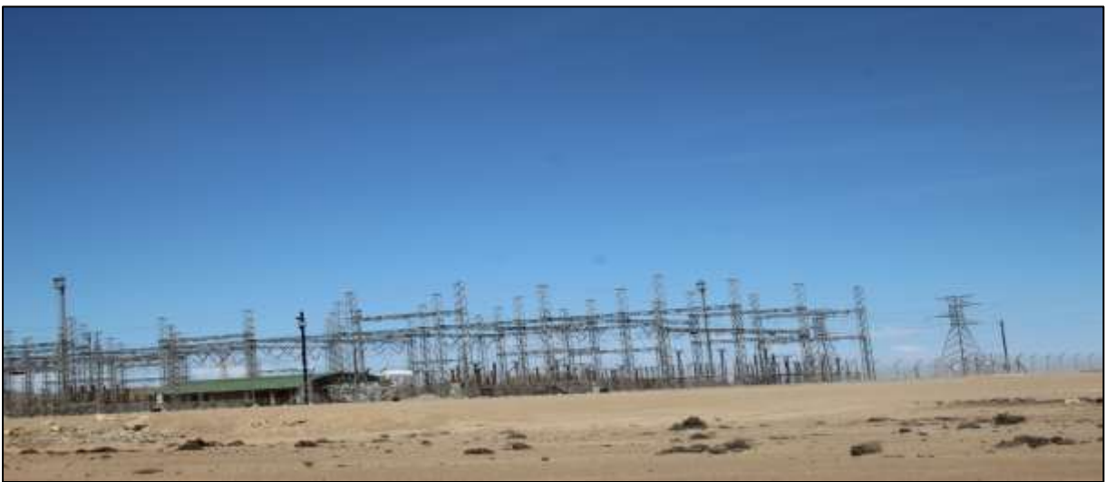
Figure 7- 2: Lithop Substation, NamPower.
