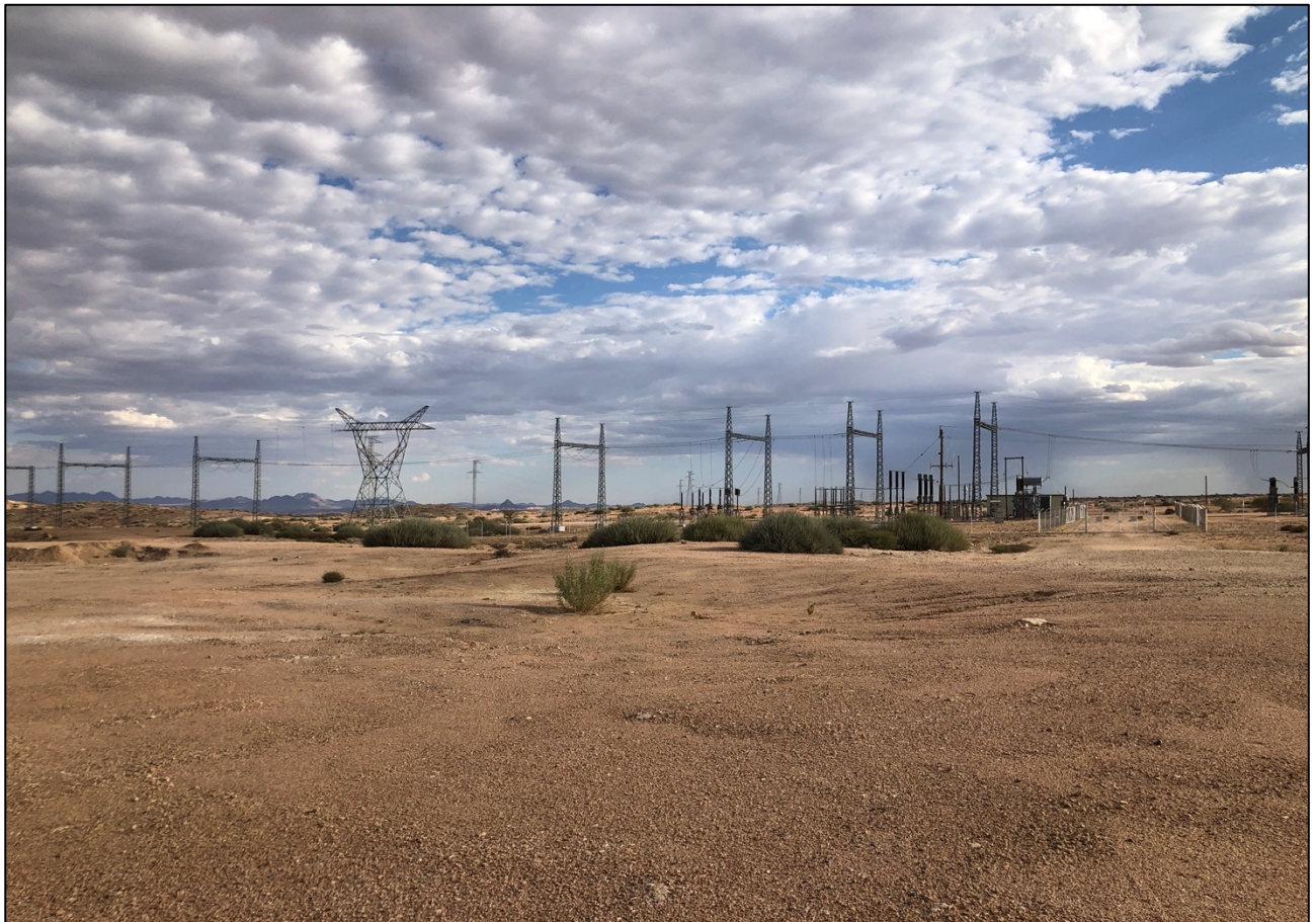
Figure 10: Existing NAMPOWER sub-station within proximity to the PV plant location
