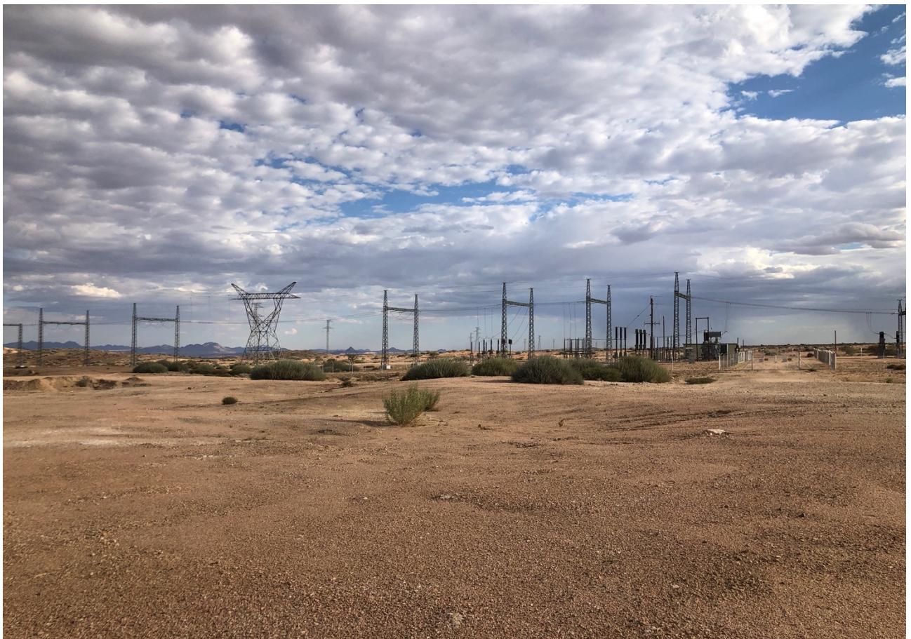
Figure 9: Existing NAMPOWER sub-station within proximity to the PV plant location
