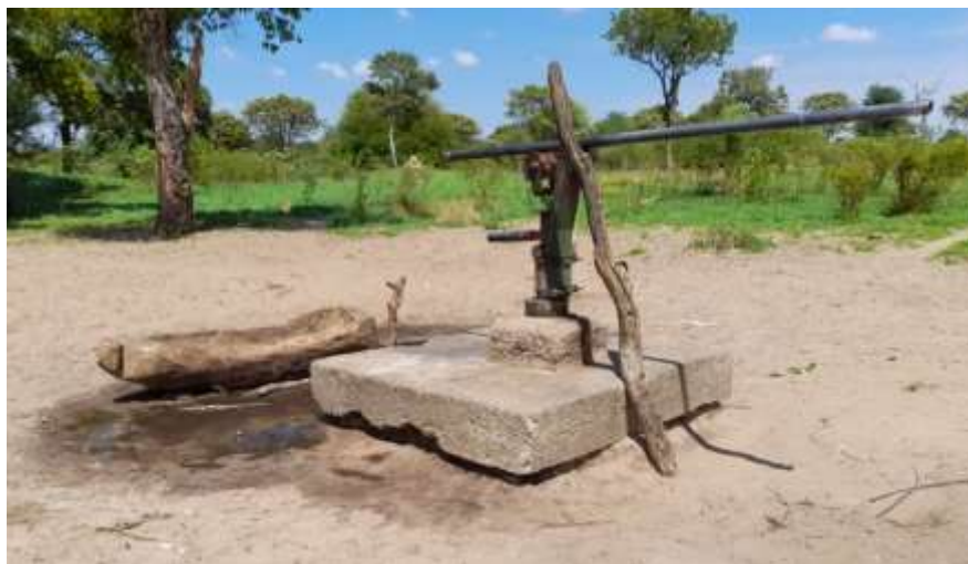
Figure 8 Hand pump water point in surrounding area
