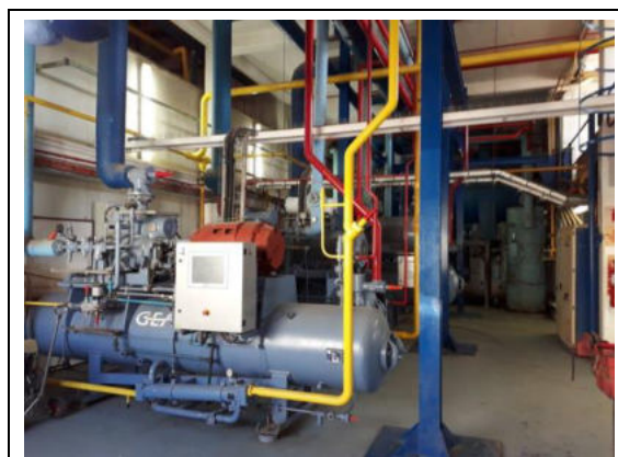
Photo 4-8 Ice plant compressor room
