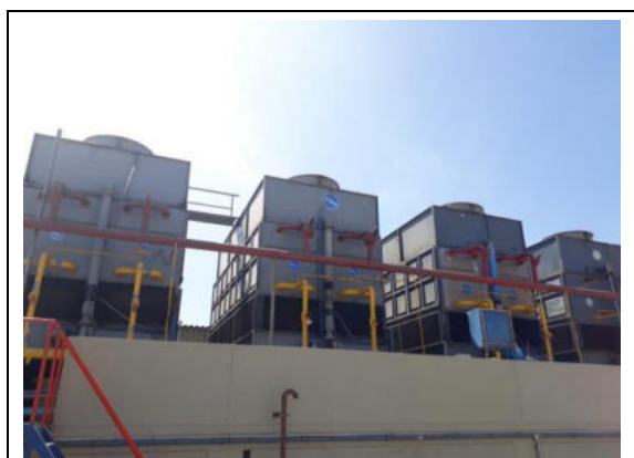
Photo 4-9 Main plant cooling towers
