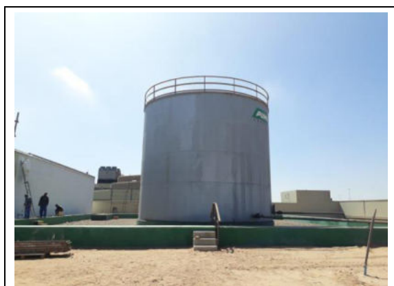
Photo 4-11 Consumer fuel installation
