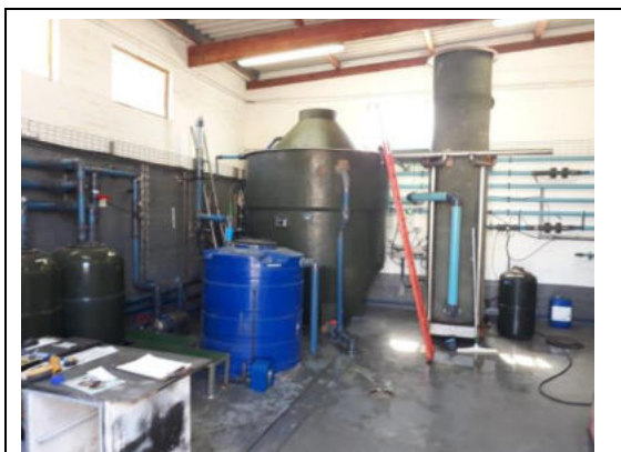
Photo 4-13 Current DAF tanks (seawater treatment)
