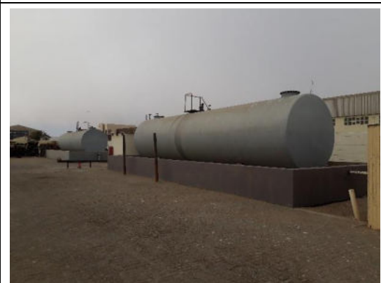
Photo 4-23 Consumer fuel installation
