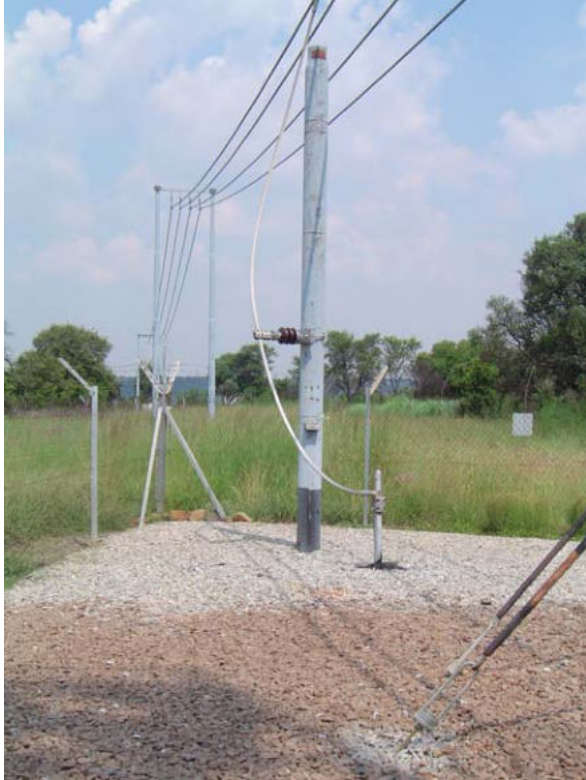
Figure 6: Earth Electrode in Fenced Off Area
