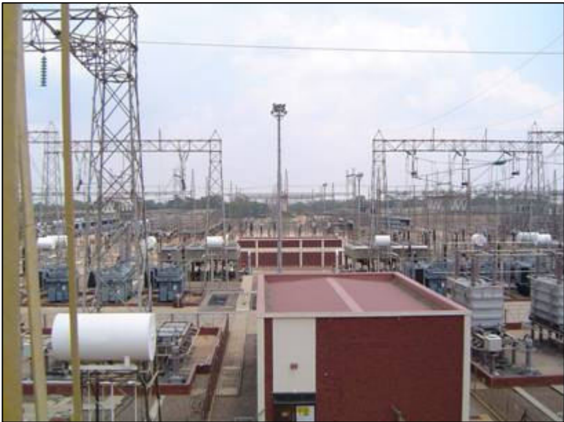
Figure 7: Typical Converter Station
