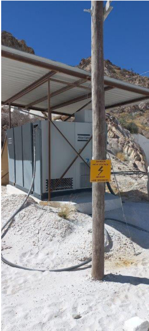
Photo 14 – View of warning sign at high voltage overhead power line and generator.
