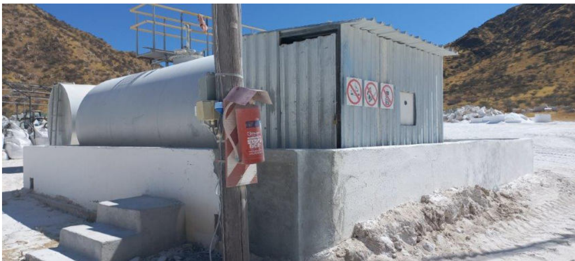
Photo 18 – View of fire extinguisher and warning signs at fuelling area.
