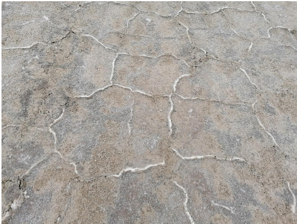
Figure 11 Salty content observed during the site visit
