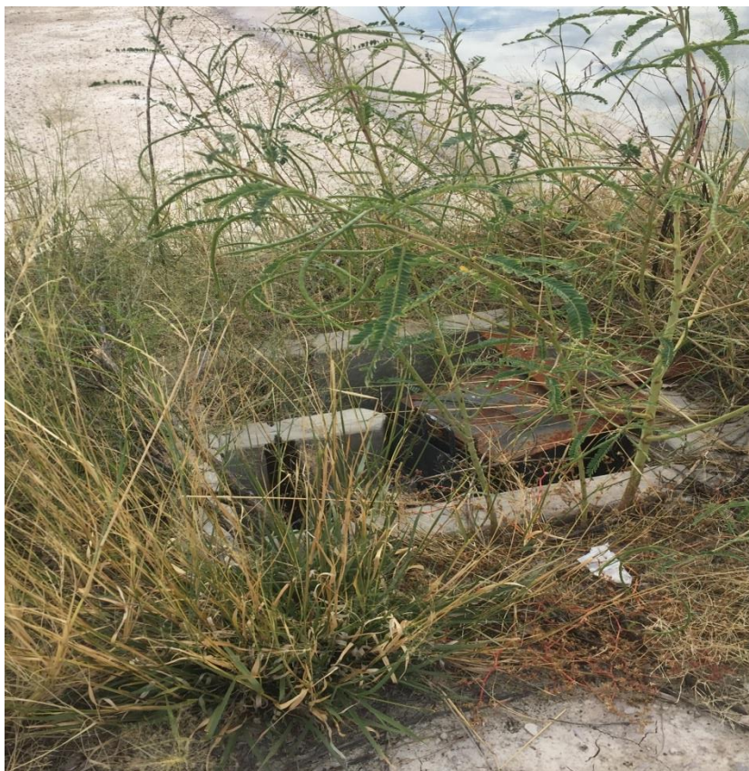
Figure 7 – Inlet structure, vegetation to be removed
