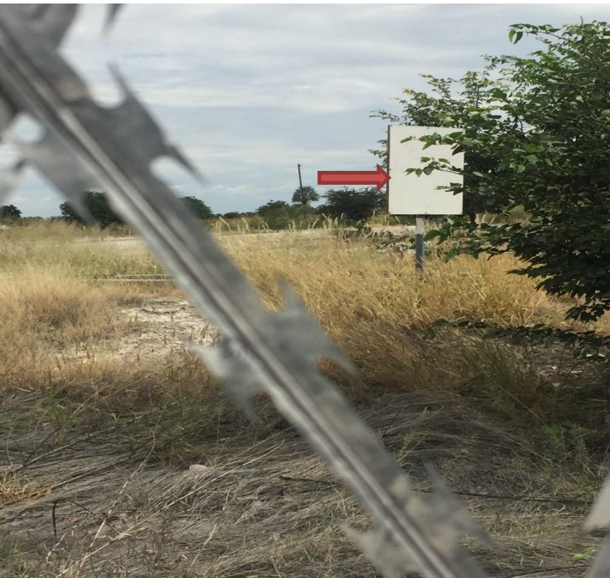
Figure 5 – Worn out warning sign that should be replaced
