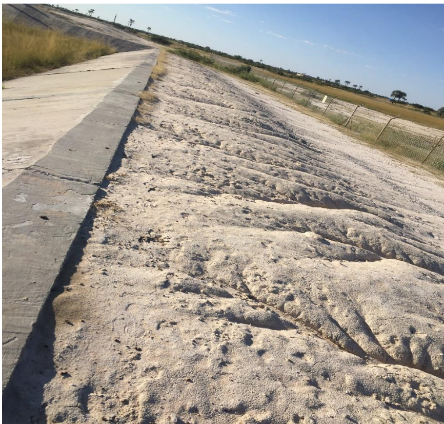
Figure 7 –Soil erosion occurring on the pond embankment walls
