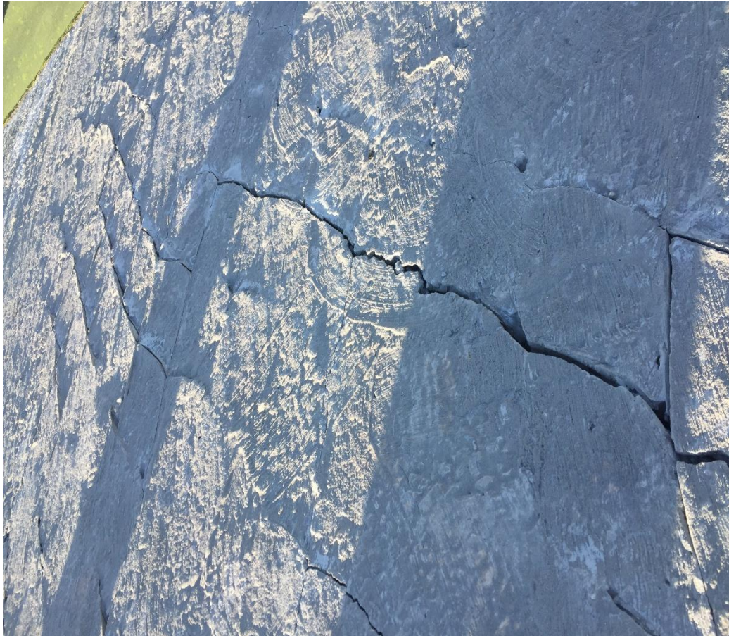
Figure 8 –Cracking on embankment concrete walls
